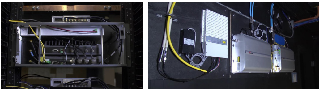
Figure 8. Example of a remote access unit
