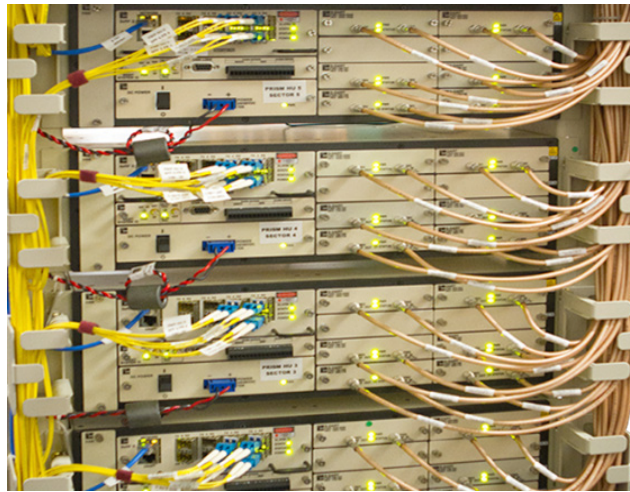
Figure 7. Example of fiber equipment at the headend
